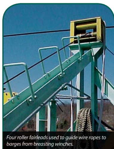
Flag type fairleads accommodate changes lead angle of wire rope as barges move.
