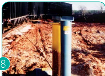
8 Railcar Puller Vertical Rope Guide & Masterlink Assembly
