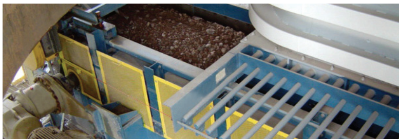
Overhead view showing an apron feeder installation under a raw mix bin at a major cement plant.
