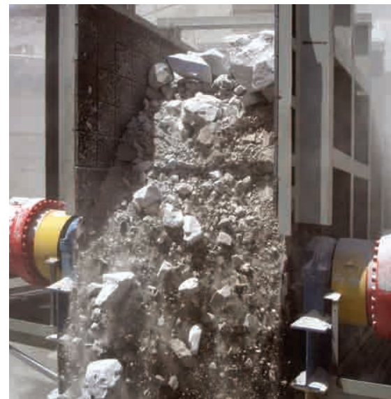
Apron Feeder extracting copper ore from a truck dump hopper to a gyratory crusher.
