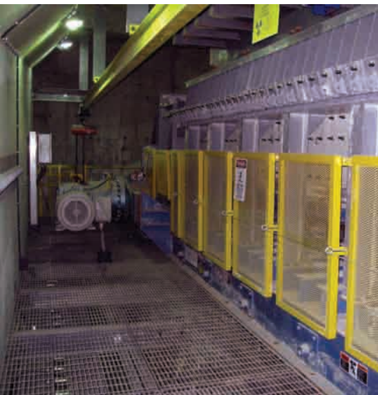
Apron Feeder installed under a crushed copper ore stockpile.
